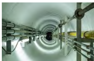
Low pressure pipelines
